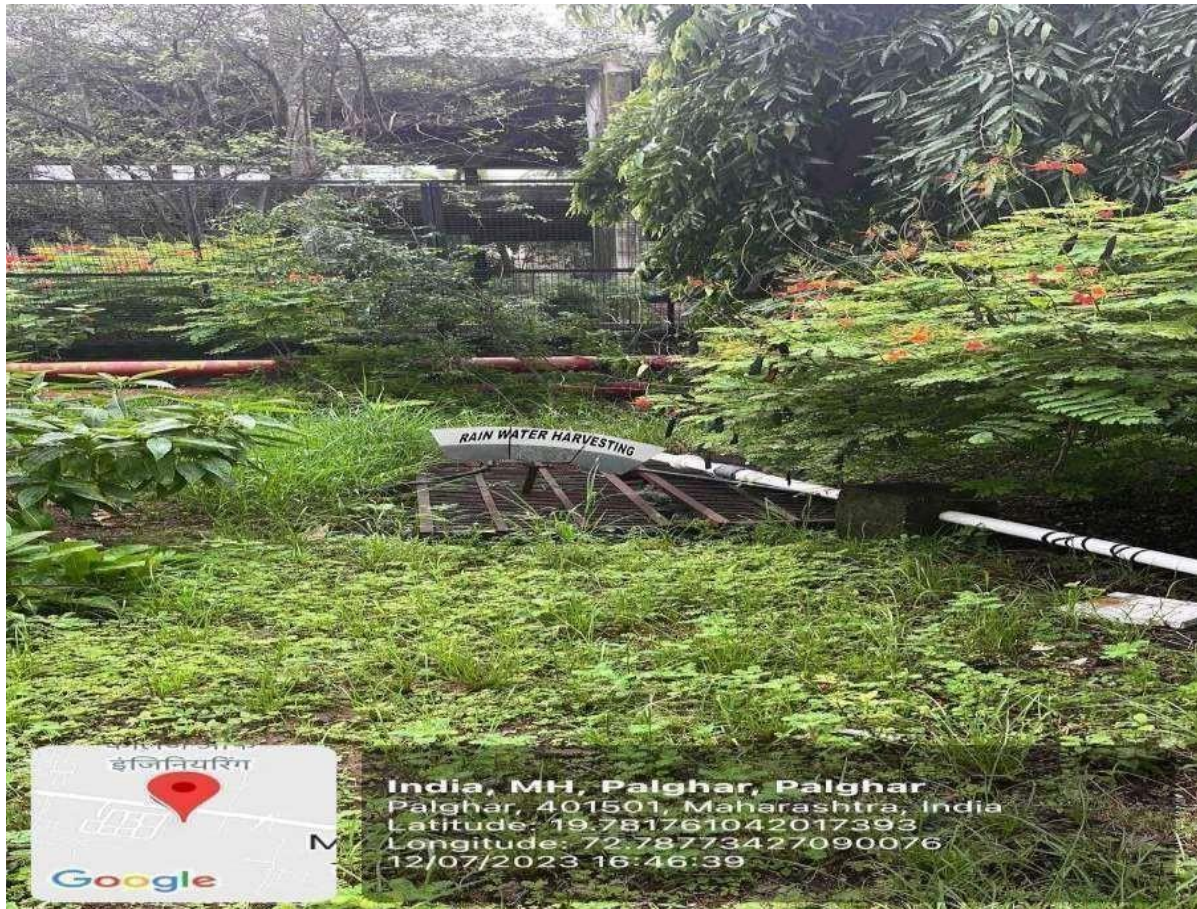
Rain Water Harvesting
