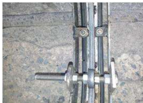
Fig.6: Support bearing mounted on M.S ring through nut and bolt and side bearing mounted on ring though nut and bolt.
