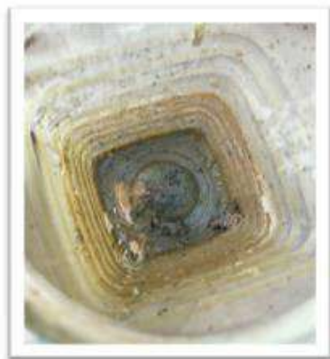
Fig. 4: Grease formation in 1 st container
